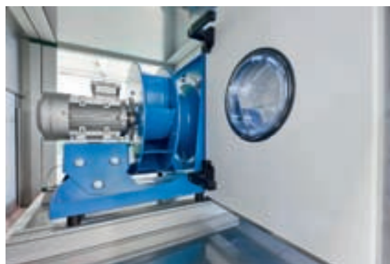
Figure 9: Plug fan and door opening inwards
